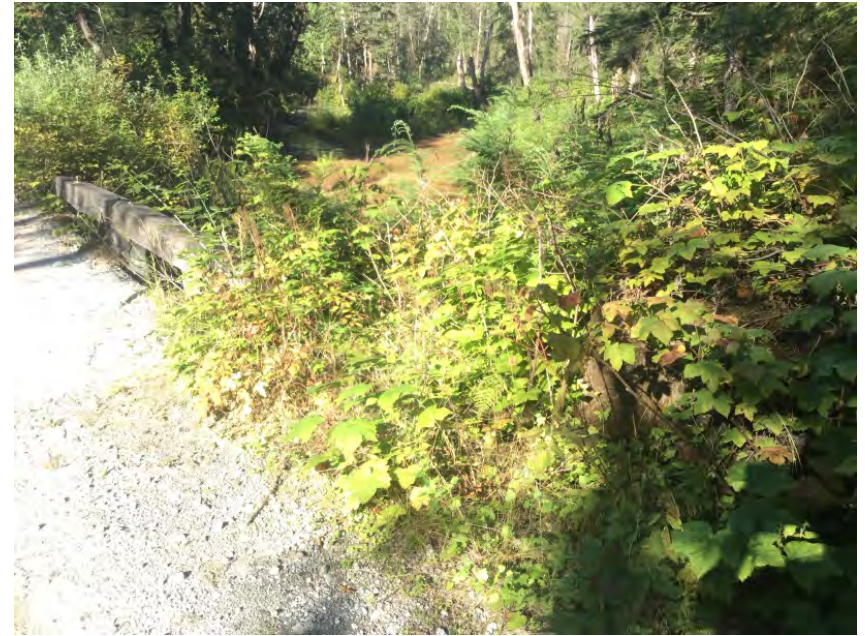
Left Approach Upstream Corner Gap between Fender & Guardrail
