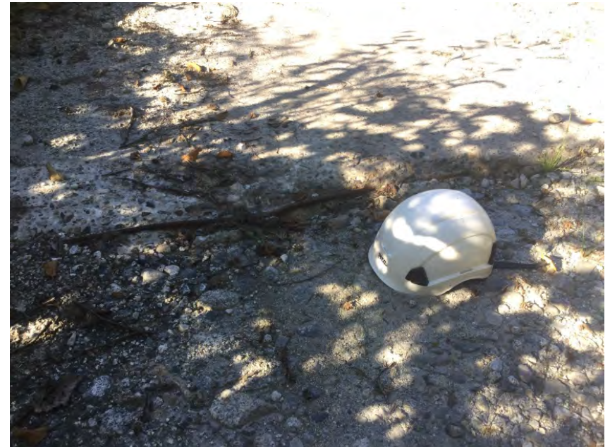
Left Approach Grade Differential & Damage to Slab
