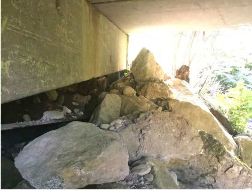
Gap between Riprap & Cap
